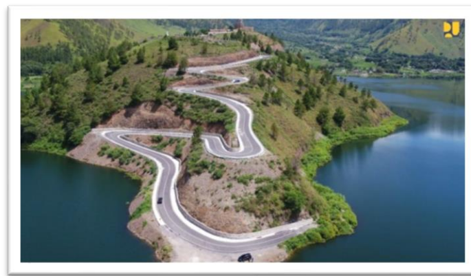
Figure 2: Construction of A Spiritual Tourism Access Road to The Jesus Statue Which Is Located on The Peak of Sibeas-Bea Hill, Samosir Regency.
